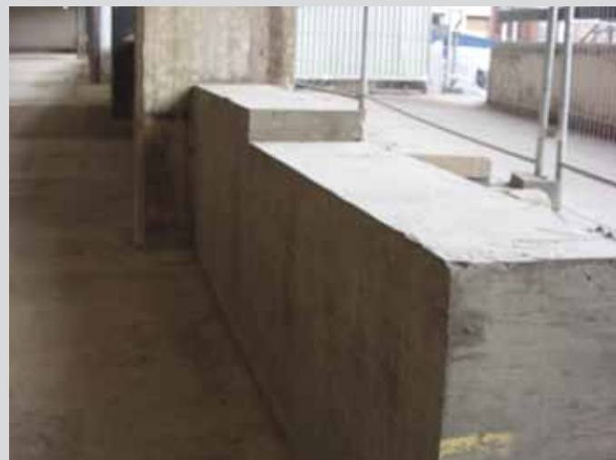
Project: Car Park Refurbishment (inc. shuttering & steelwork for concrete upstand) Main Contractor: PBM Building Services Ltd Contract Value: £120,000 Year: 2009
