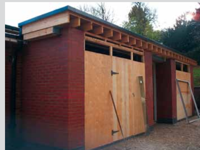
Project: Sheffield Children's Centres Main Contractor: Kier Sheffield LLC Contract Value: £200,000 Year: 2007
