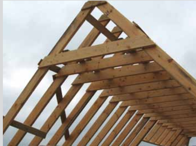
Project: Housing Traditional Roof Construction Main Contractor: Private Client Contract Value: £170,000 Year: 2007/2008
