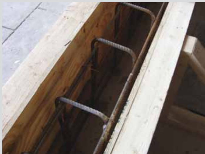
Project: Car Park Refurbishment (inc. shuttering & steelwork for concrete upstand) Main Contractor: PBM Building Services Ltd Contract Value: £120,000 Year: 2009
