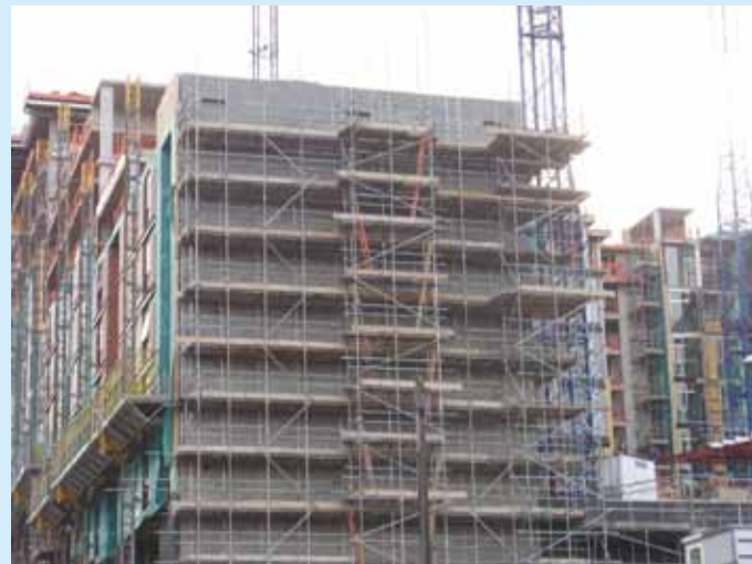
Project: Gateway Plaza (Barnsley) Main Contractor: Browns Construction Group Contract Value: £600,000 Year: 2008 / 2009
